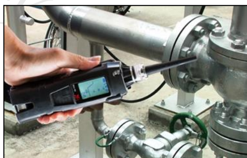
For gas pipe joint
